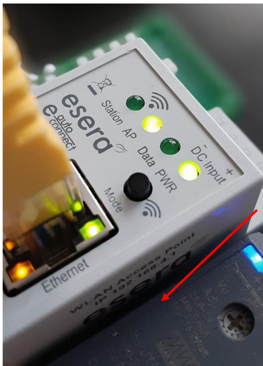
Access Point is activated
